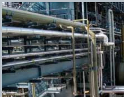
GRP piping, part of a chemical processing plant
