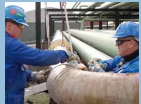
The lamination of a GRP pipe for chlorine gas by our well experienced installation personnel
