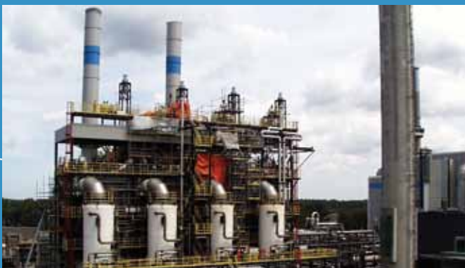
GRP covers, tanks and ducts in a waste incineration plant
