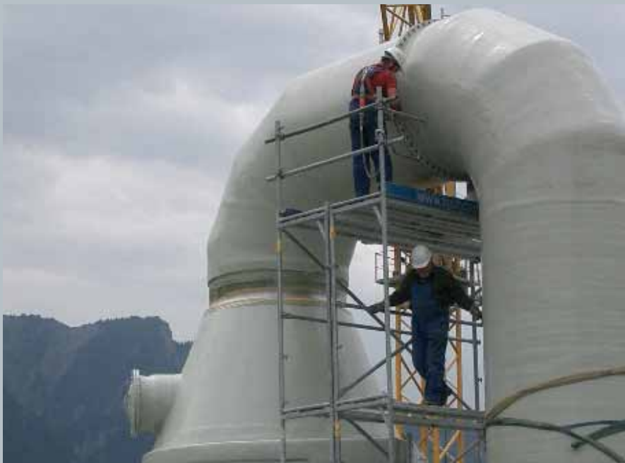
GRP piping, installed by our installation people
