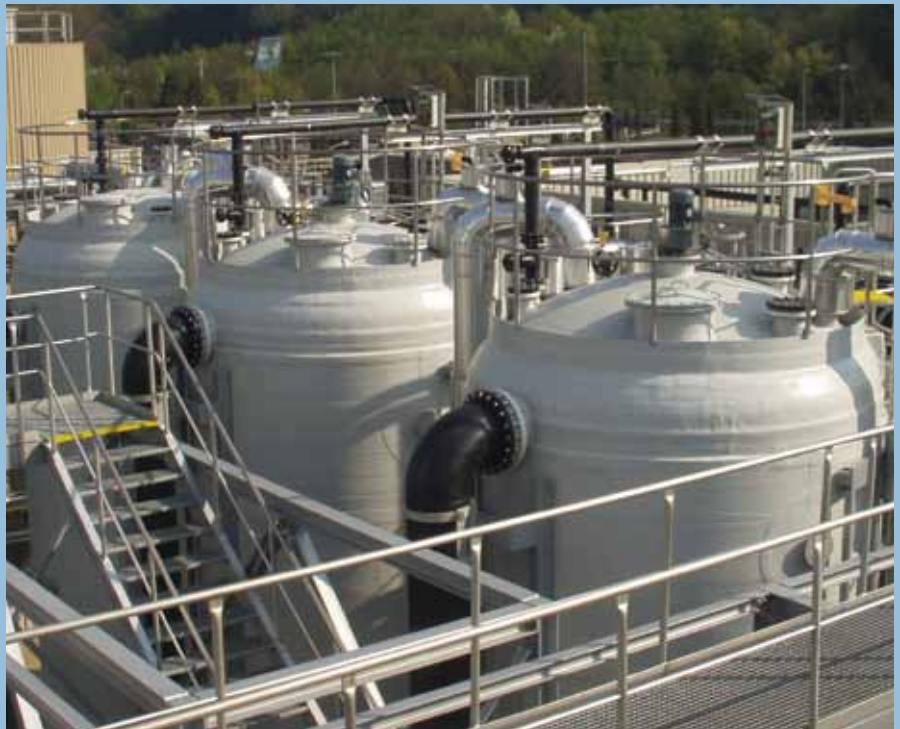
Storage of waste water at 90 °C (3 x 120 m 3 , D = 3500 mm)
