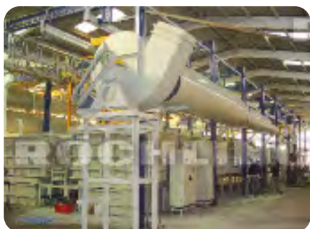
Polystone® P homopolymer grey Ventilation system for a galvanic plant
