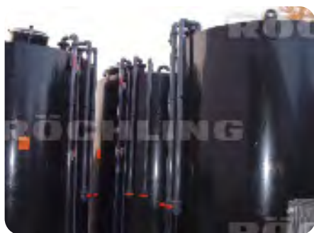
Polystone® G black B 100 Storage tanks for sulfuric acid
