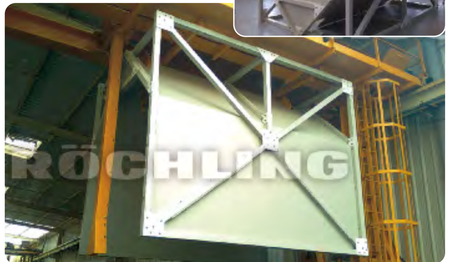
Foamlite® P grey Mobile hub of a galvanic line (installed)
