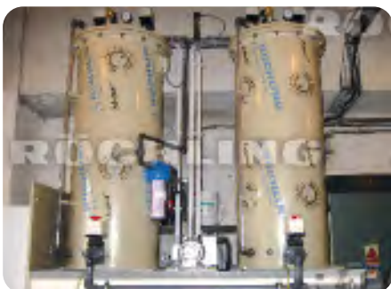
Polystone® P homopolymer grey Exhaust-air scrubber
