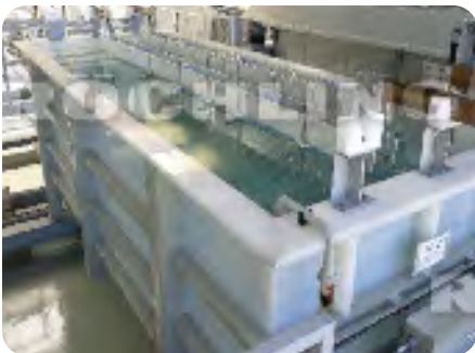
Polystone® P homopolymer natural Anodisation basin for treating door handles
