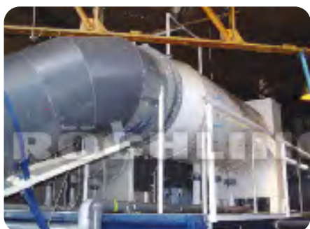
Trovidur® EC and Polystone® PVDF Ventilation plant
