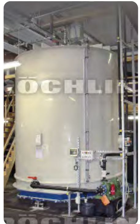
Polystone® P homopolymer grey Mixing tank with a capacity of 25 m 3
