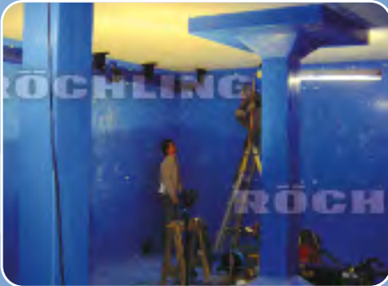
Polystone® G HD blue Lining of a drinking-water reservoir
