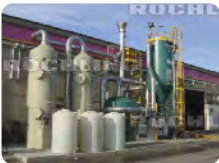
Polystone® P copolymer grey Exhaust-air treatment facility for odour elimination
