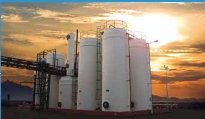
Storage solution (20 – 150 m 3 ) at a fertilizer plant
