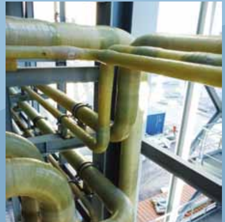
GRP piping, part of the chemical processing at a steel plant
