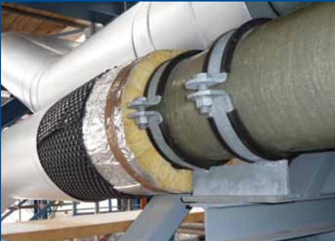
Insulation (50 mm rockwool) and supporting of a pipeline in a chlorine plant
