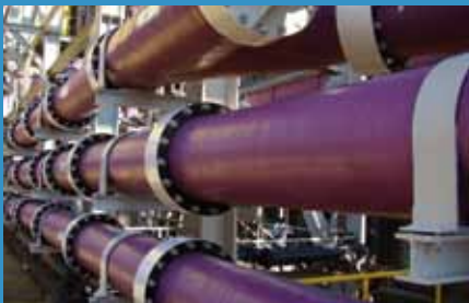
PVC/GRP pipes for the transport of Hydrochloric acid (30%) at 60°C
