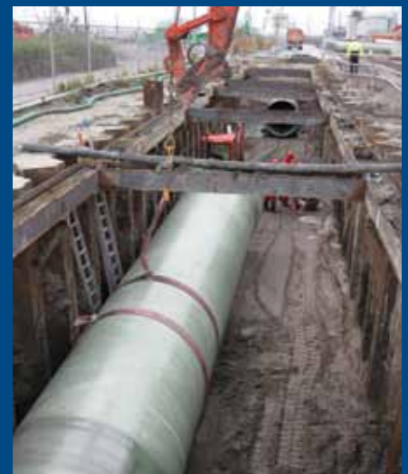
The installation of an underground cooling water pipe (D = 1600 mm) at a coal fired power plant
