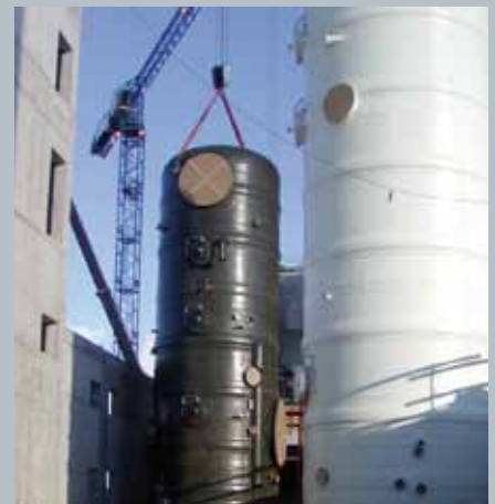
A scrubber of D = 3.5 meter cleaning Hydrochloride acid gasses
