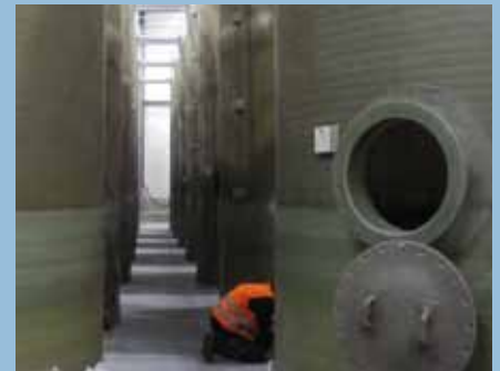
Inspection opening D = 800 mm in large diameter tanks
