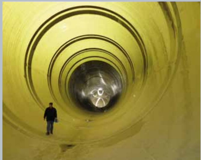
Inspection of a 10 meter diameter duct by our well experienced QA personnel
