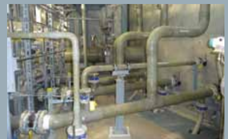
GRP piping at a power plant in Germany
