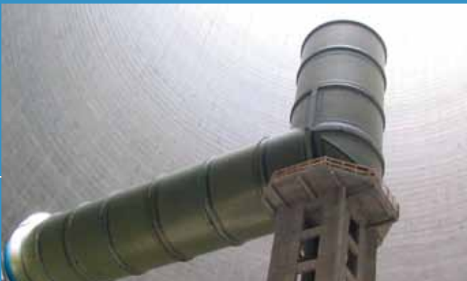
Duct D = 10 meter, L = 150 meter in a cooling tower at a coal fired power plant
