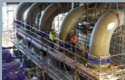
Quality inspection of GRP recirculation piping on an absorber (D = 1200 mm, P = 10 bar)
