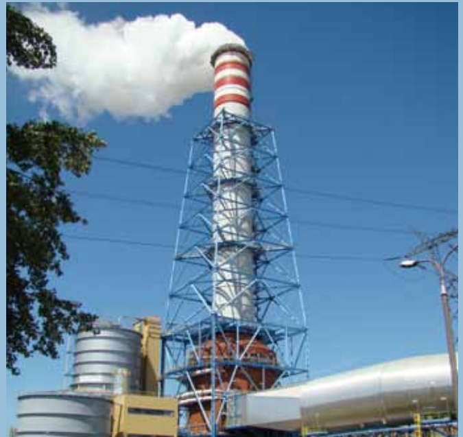
A steel supported GRP stack of 10.2 meter on top of an absorber
