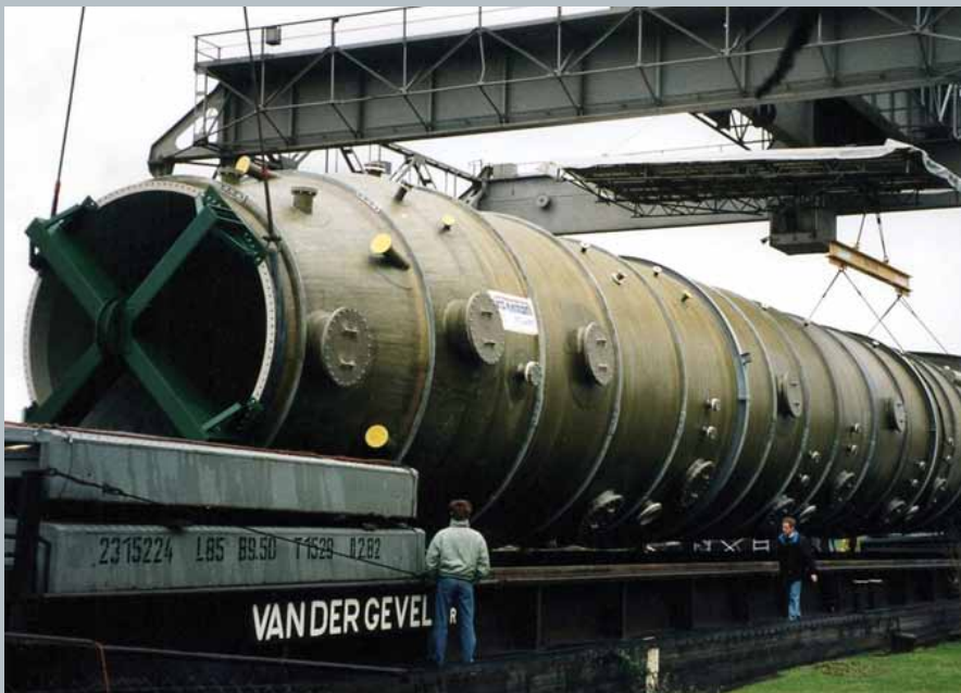
Lifting of a scrubber of D = 5 meter, H = 30 meter for an waste incineration Plant in Germany
